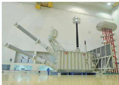
±1100kV Converter transformer
