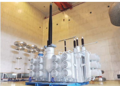
1000kV AC transformer
