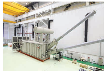
±800kV Converter transformer
