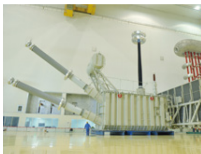
采用B23R075制造的±1100kV特高压换流变压器性能 The performance of the ±1100kV UHV converter transformer made with B23R075
