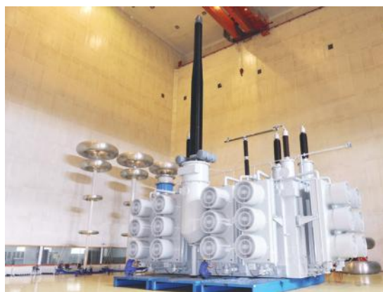
采用B27R090试制的双百万变压器性能 Properties of the dual million transformer made of B27R090
